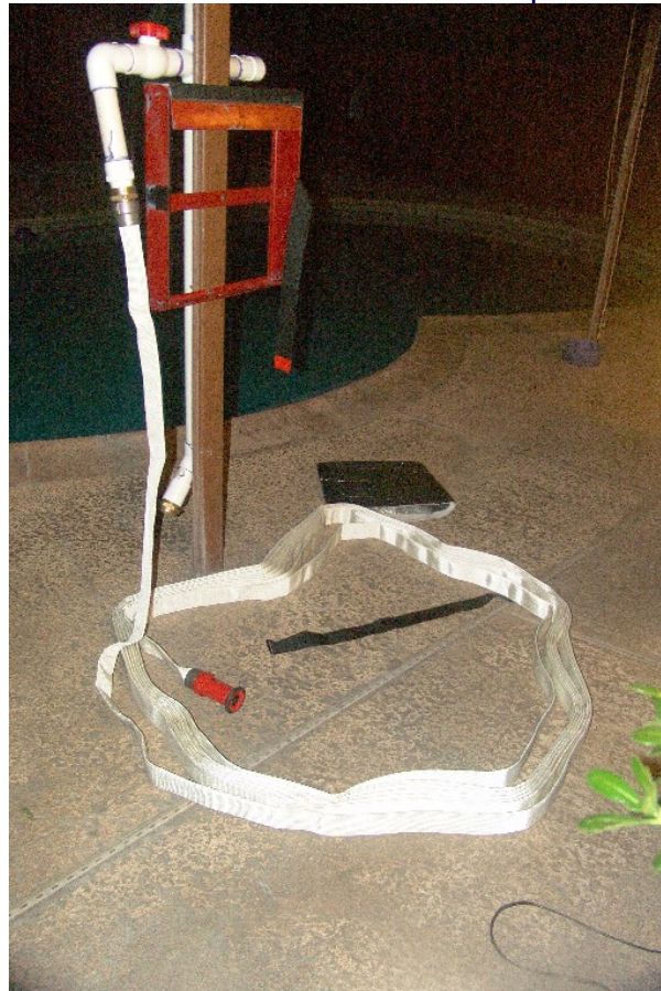
The hose is now FIRE READY for FULL water pressure
